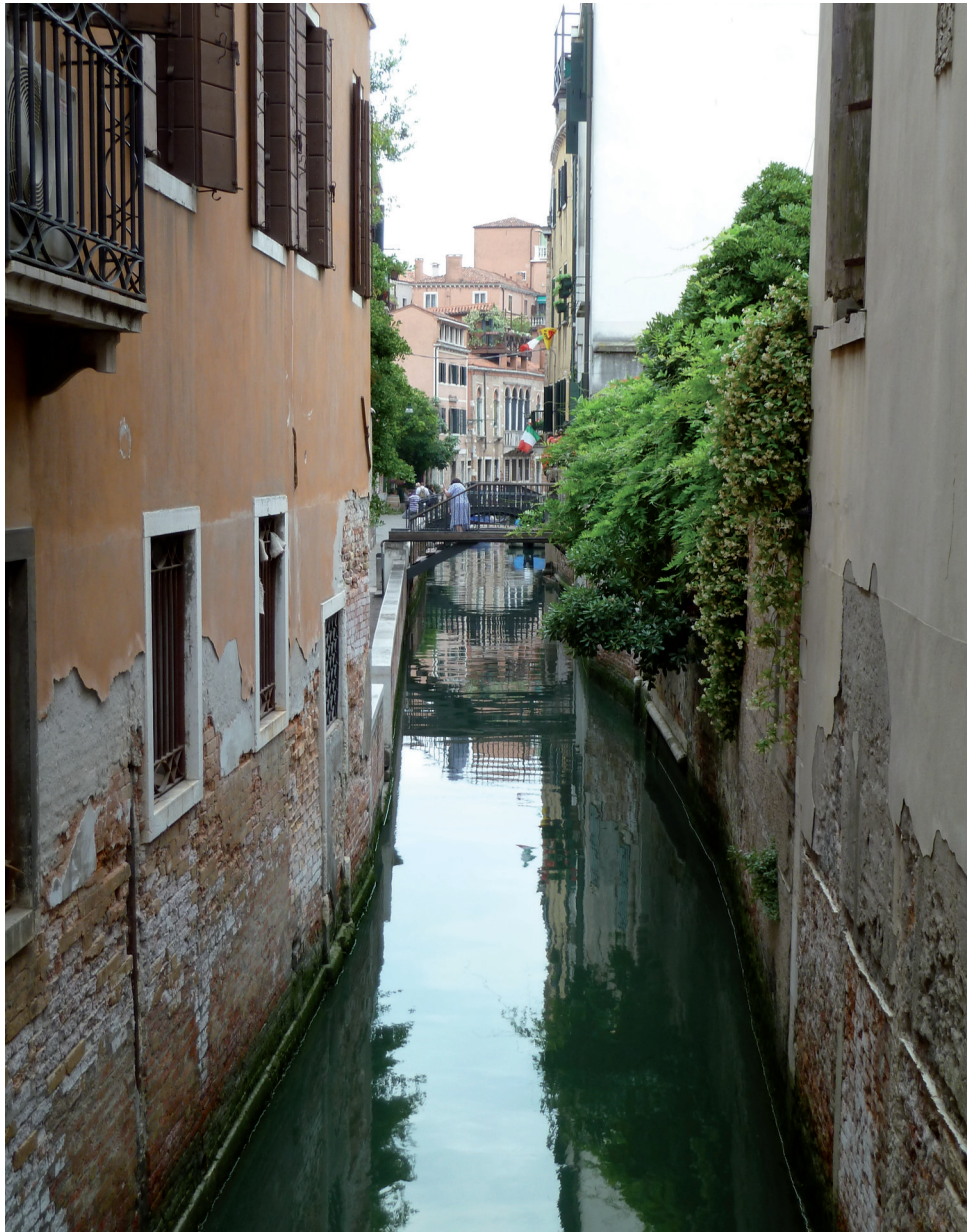
© Abxbay - Rising damp damage to brickwork and masonry, Rio de la Frescada
